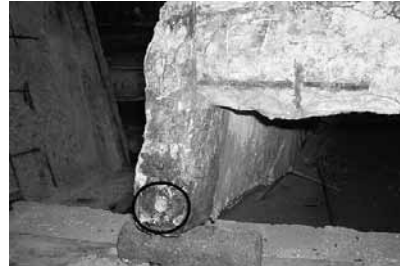
Fig. 4. The support of panel R7 after anchorage failure.
