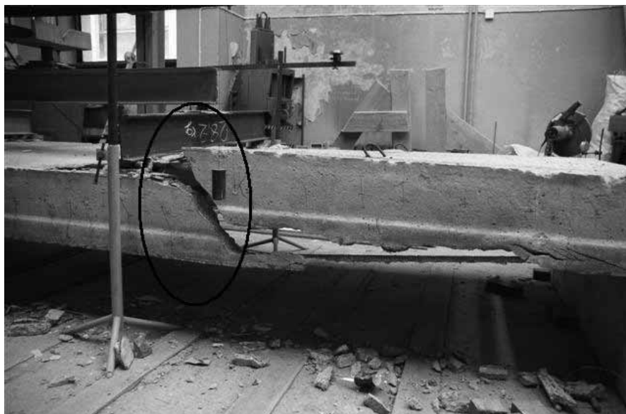
Fig. 4.9. Shear failure of ribbed panel V12.
