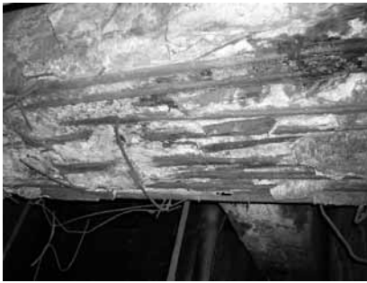
Fig. 2. Bottom view of a girder fragment carrying generator on the 2nd floor.
