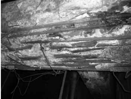
Fig. 4.11. Bottom view of a fragment of a girder carrying a generator on the 2nd floor.
