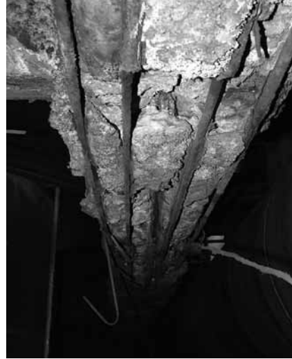
Fig. 4.12. Bottom view of a fragment of a joist carrying a generator on the 2nd floor.
