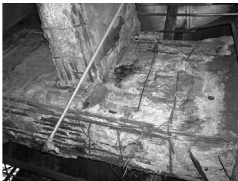
Figure 2. Condition of some concrete beams on the first floor
